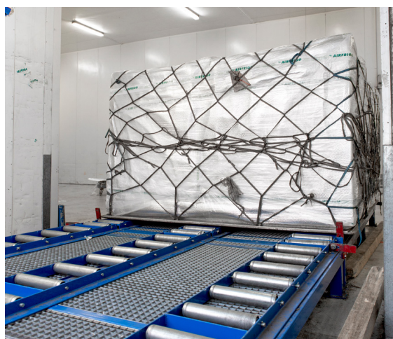
Cold storage © Seafrigo
